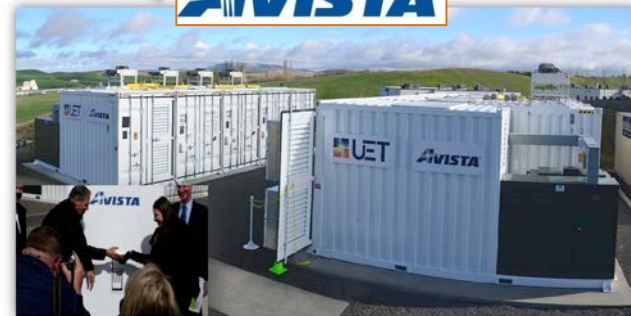
1 MW/3.2 MWh UET vanadium-flow battery Pullman, WA
